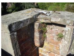
Fractured capping stone
