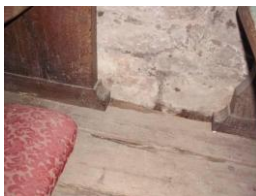
Low level damp
